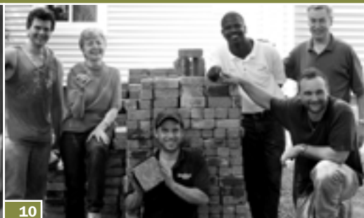
Volunteers from Ridgewood A.M. Rotary and the NJ Landscape Contractors Association build a patio for the little girls.
